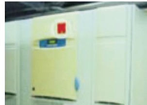
UPS房溫度偵側
